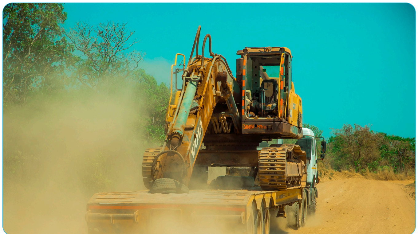
Road works in Katavi Region, similar to what the Government has set aside for local contractors
